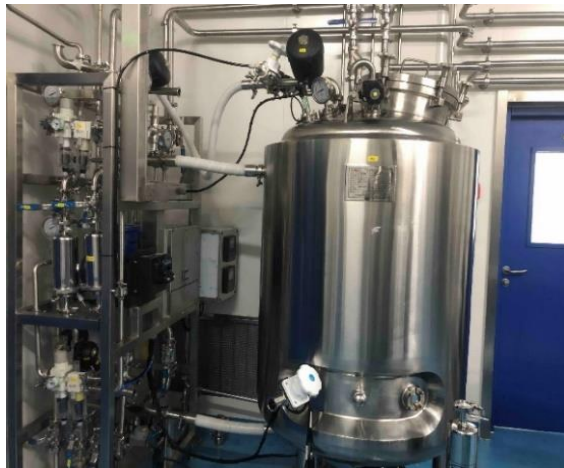
Explosion Proof Facilities/ High-potency Suite
