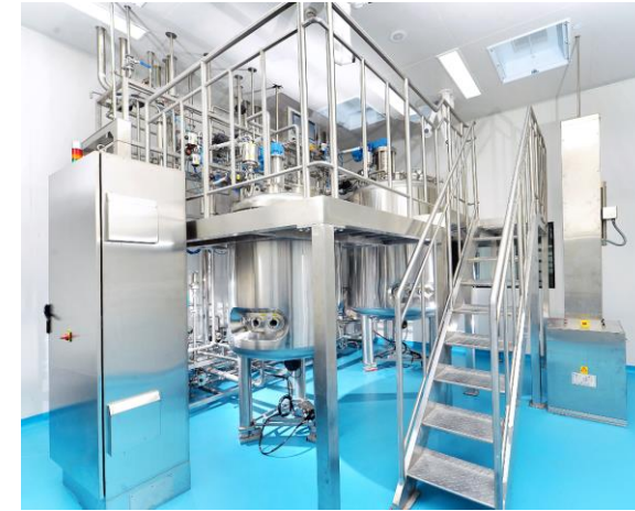
Automatic buffer Configuration/storage system
